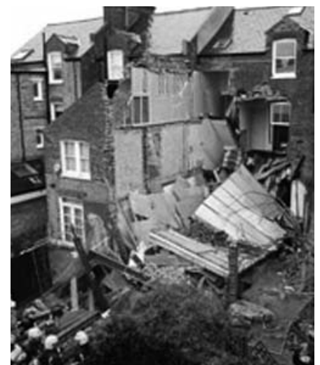
Battersea house collapse
