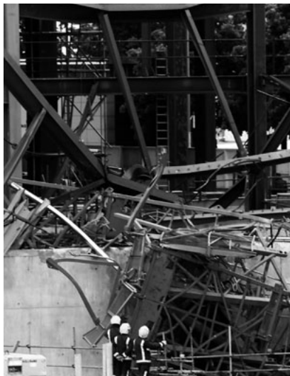
Collapsed crane at canary wharf
