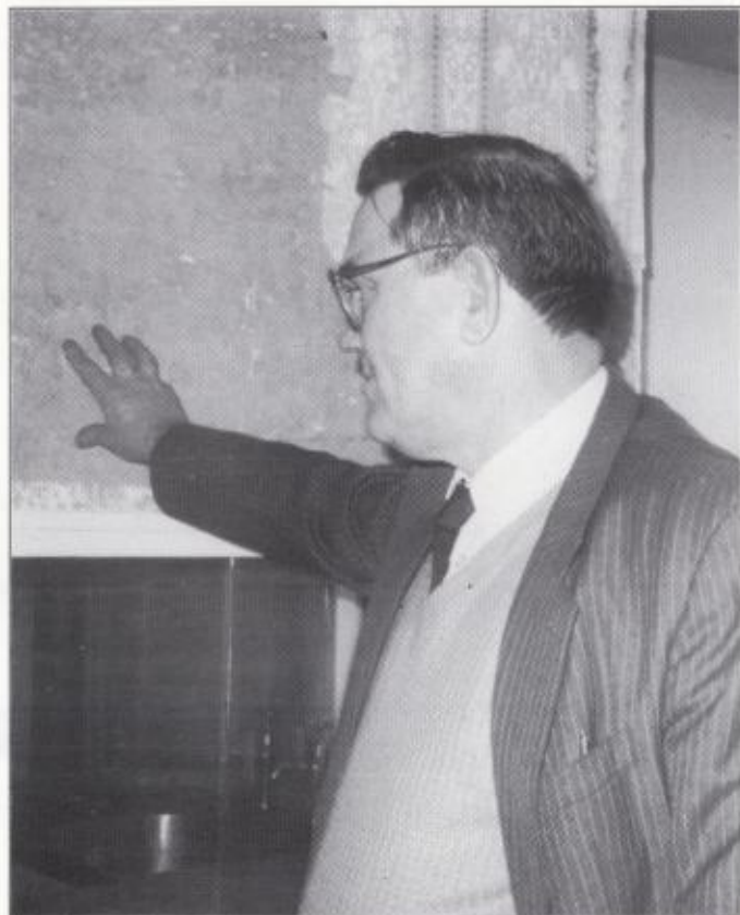
Len Fay, Chair of the Tenants Association, points out a typical asbestos wall in an empty, vandalised flat.
