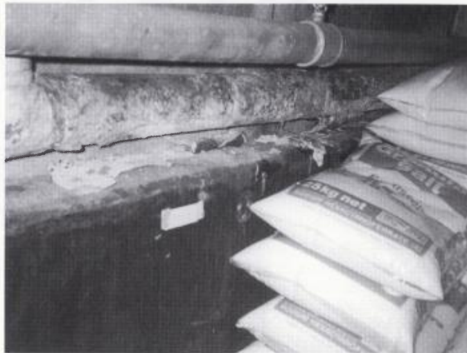
Asbestos insulation in poor condition (missed by survey)
